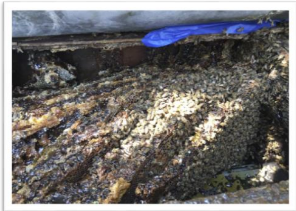
Memorial Gym Roof –Honey Bee colony A Honey Bee colony was discovered during construction and was removed/relocated
