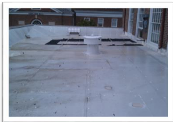
Peabody Hall Roof - Before
