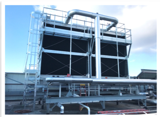
Aurbach – Cooling tower after
