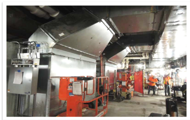
Chemistry – New AHU's 201 & 502
