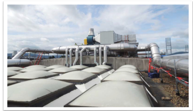
Chemistry – New exhaust fan & energy recovery
