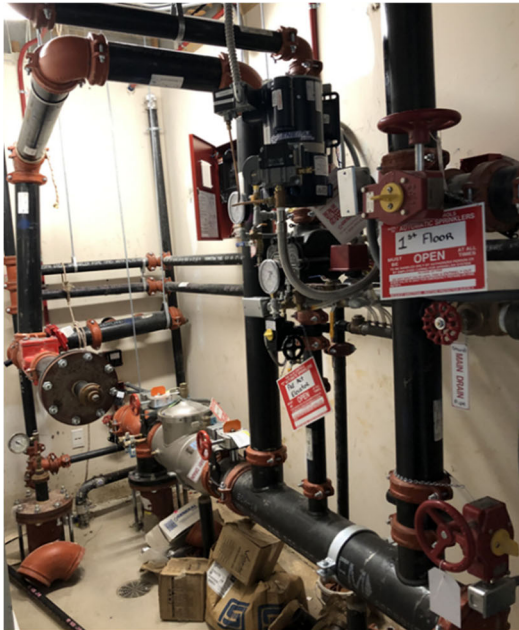
Michie Building – Newly installed suppression infrastructure
