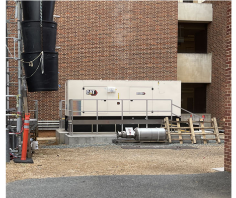
Chemistry Addition – New generator
