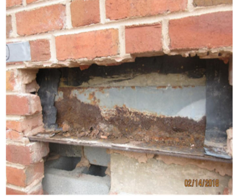
North Chiller Plant – Example of failing shelf angle
