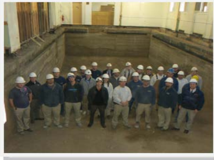
Rugby – Debris removed from pool
