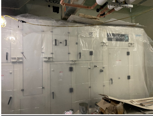
New mechanical unit on Level 2 existing building.
