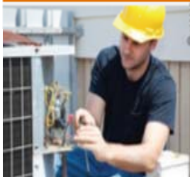
UVA Employees are never allowed to work on energized equipment
