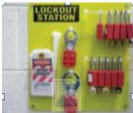
Ensure you have the proper tools to properly perform a lockout-tagout
