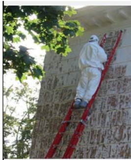
Wet scraping (removal of loose and flaking paint) performed by a licensed de-leading contractor
