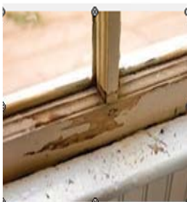
Flaking paint on a windows sill: assume it contains lead paint unless testing indicates otherwise
