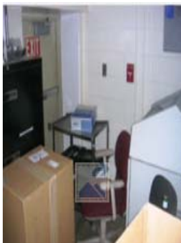
Ensure boxes/materials are not blocking egress route
