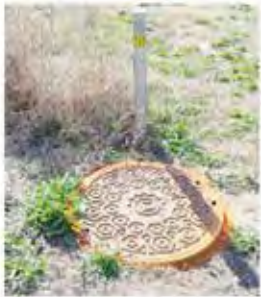
Manhole cover marking
