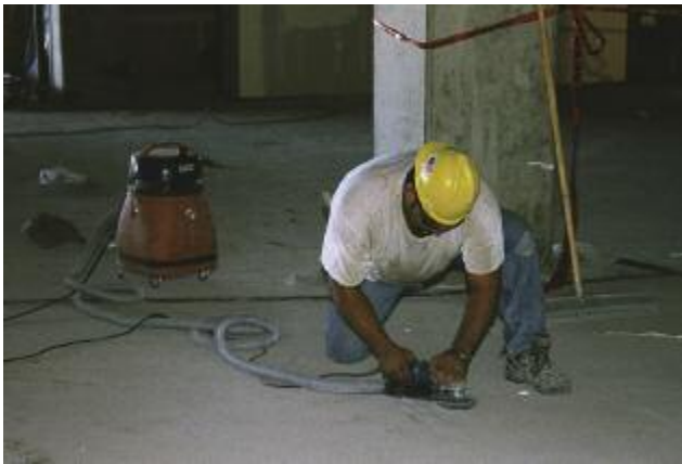
Grinder with attached VDC system. (Photo courtesy of the University of Washington.)
