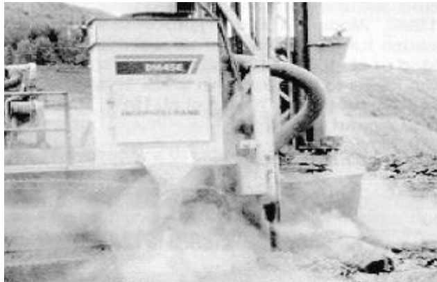
Earth drilling rigs operated without dust controls are capable of producing very high respirable silica levels (Photo courtesy of NIOSH, 1992.)
